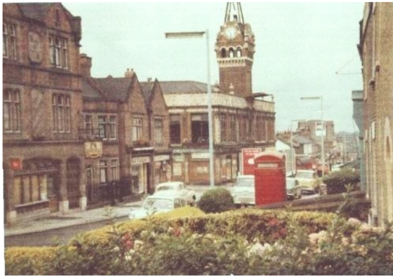
The R.A.C.S. Department Co-op store in the process of being demolished with its clock tower spire roof removed.
